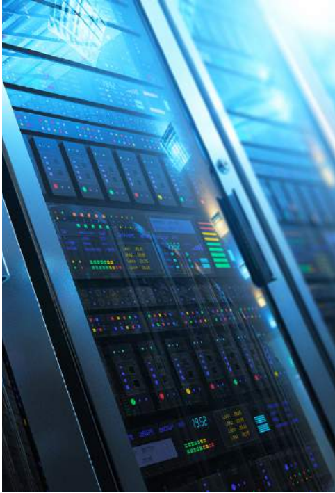
AI High Performance Data Center
