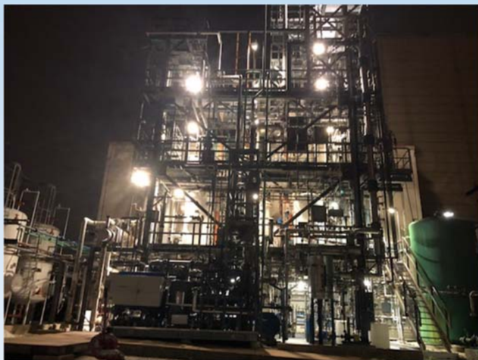
New LED lighting courtesy of the Appleton Group
