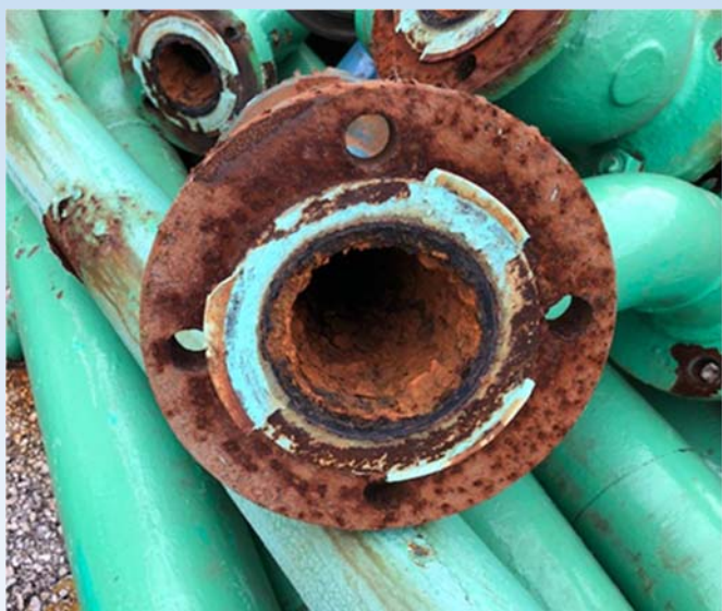
Original Carbon Steel Cooling Water Piping
