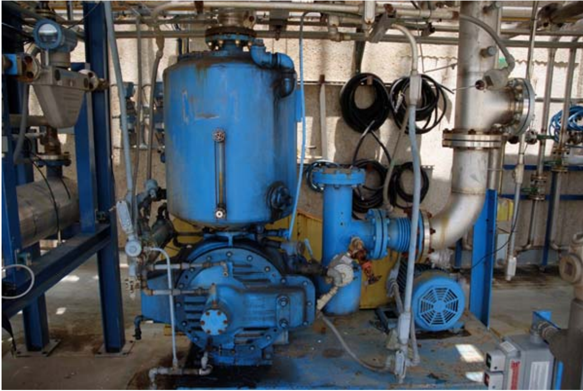
Figure 1-5. Vacuum Pump (C-102A) Draws Gas from the Right Side and Discharges from the Top of the Oil Reservoir (Picture Taken by C. Lewis)
