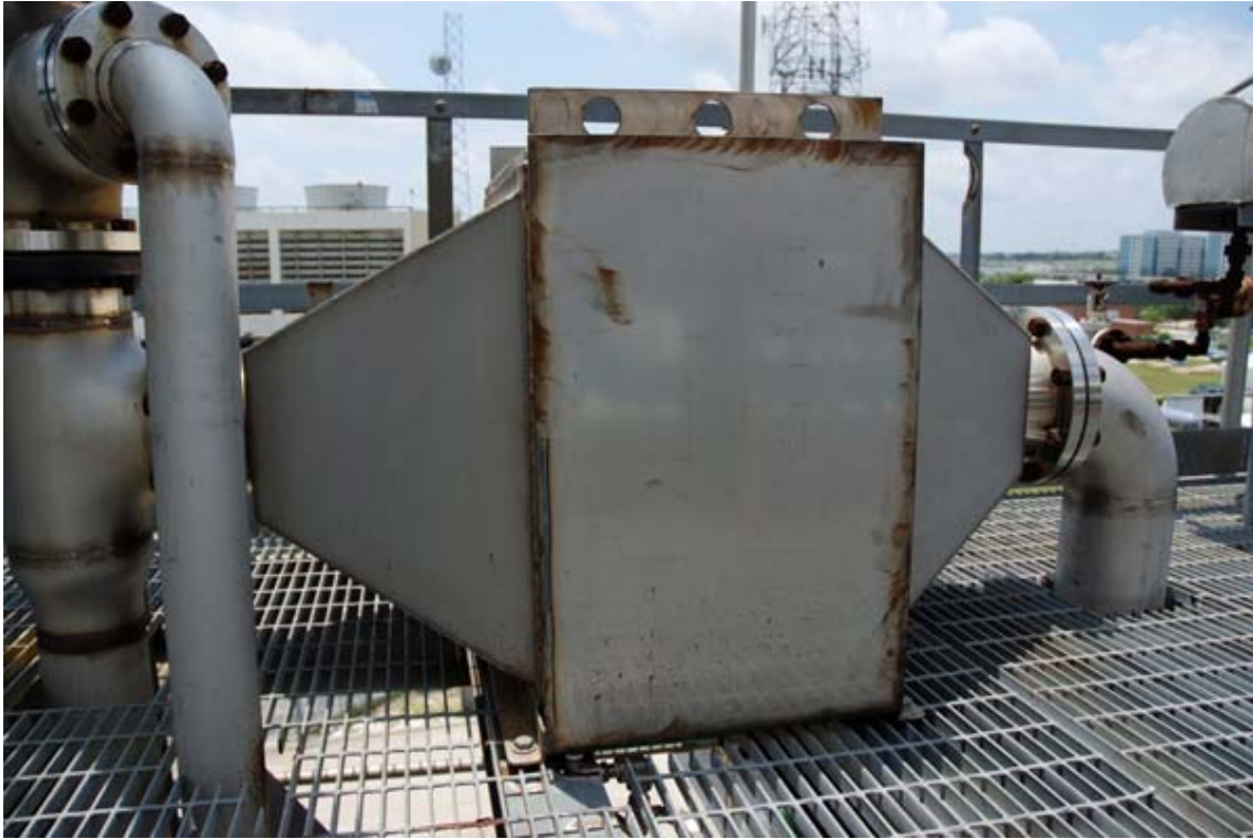
Figure 1-8. Air Cooler (H-112) as Installed on Top Platform of Structure. Radiator Coils are Located on the Opposite Side (Picture Taken by C. Lewis)
