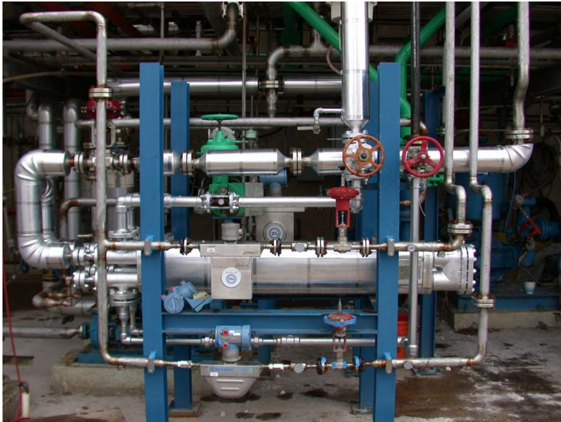
Figure 1-6. Solvent Preheater (H-101A & B) as Installed on Support Rack, along with Micro Motion ® Flowmeters, and Control Valves (Picture Taken by C. Lewis)
