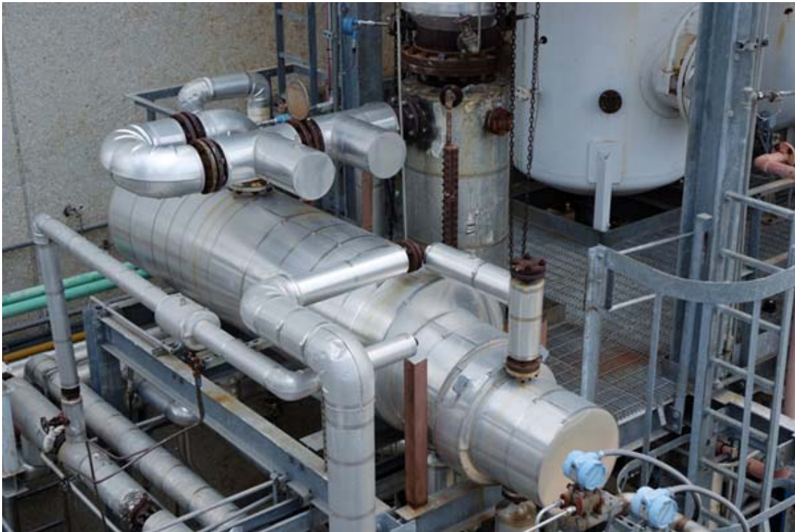
Figure 1-24. Stainless Reboiler and Stripper Column Sump with Calcium Silicate Insulation
