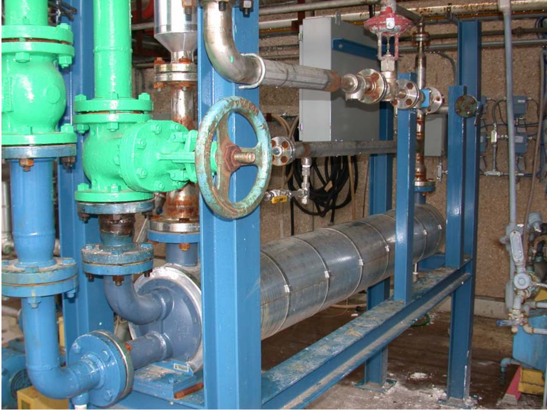
Figure 1-7. Solvent Cooler (H-107) as Installed on Support Rack. Cooling Water Piping is Painted Green and Flows Tubeside (Picture Taken by C. Lewis)
