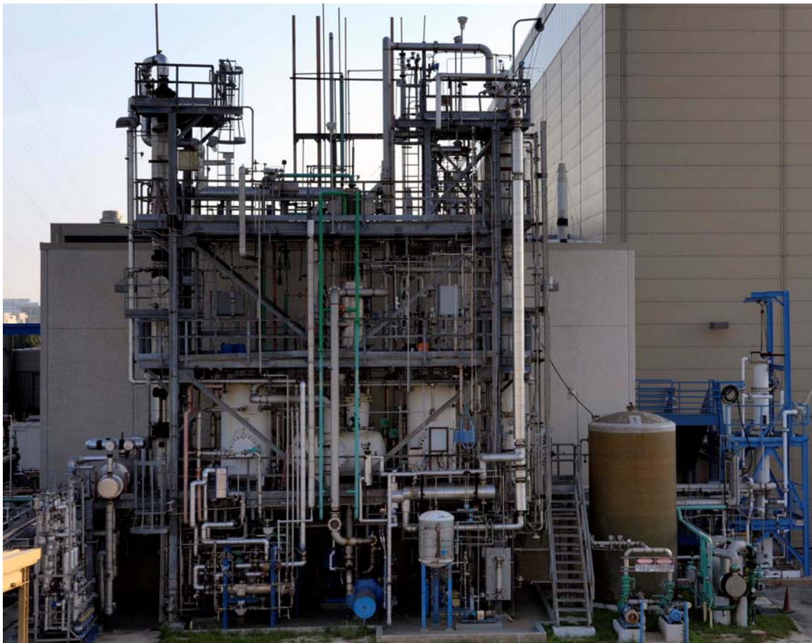
Figure 1-1. Pilot Plant Facility Located at UT SRP with the Stripper Column and Reboiler on the Left Side, Absorber Column on the Right Side, Absorber Feedtank and Overhead Gas Accumulator on the First Platform (Picture Taken by C. Lewis)
