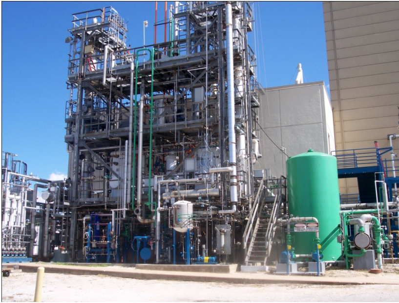
Figure 1. SRP CO 2 capture pilot plant
