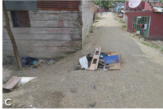
C Orificio para desaguar realizado por los vecinos. A new drain to address flooding installed by residents.
