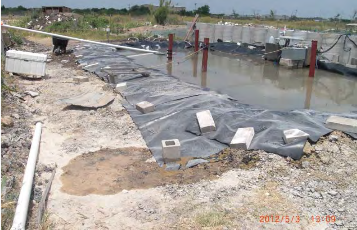
Figure 4.36: Leakage from southeast corner of inundation zone.
