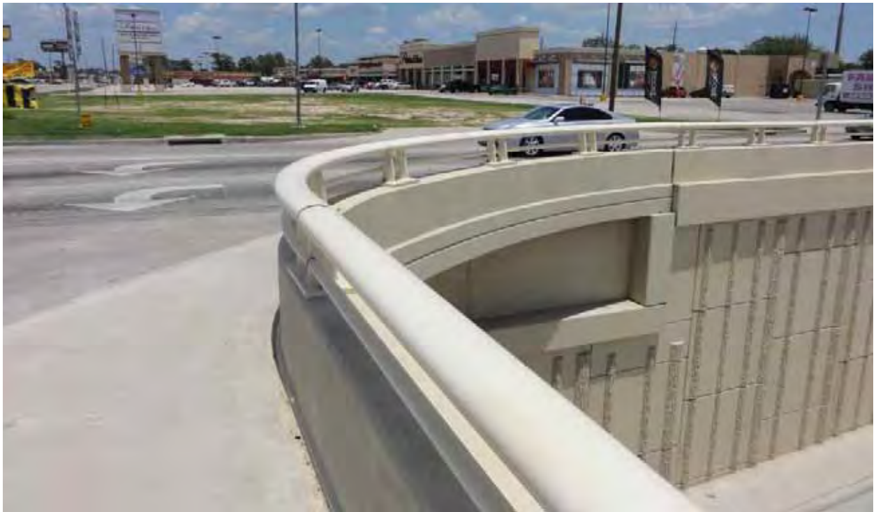
Figure 3.29: View of nearest location for moisture infiltration, at southeast corner of intersection.
