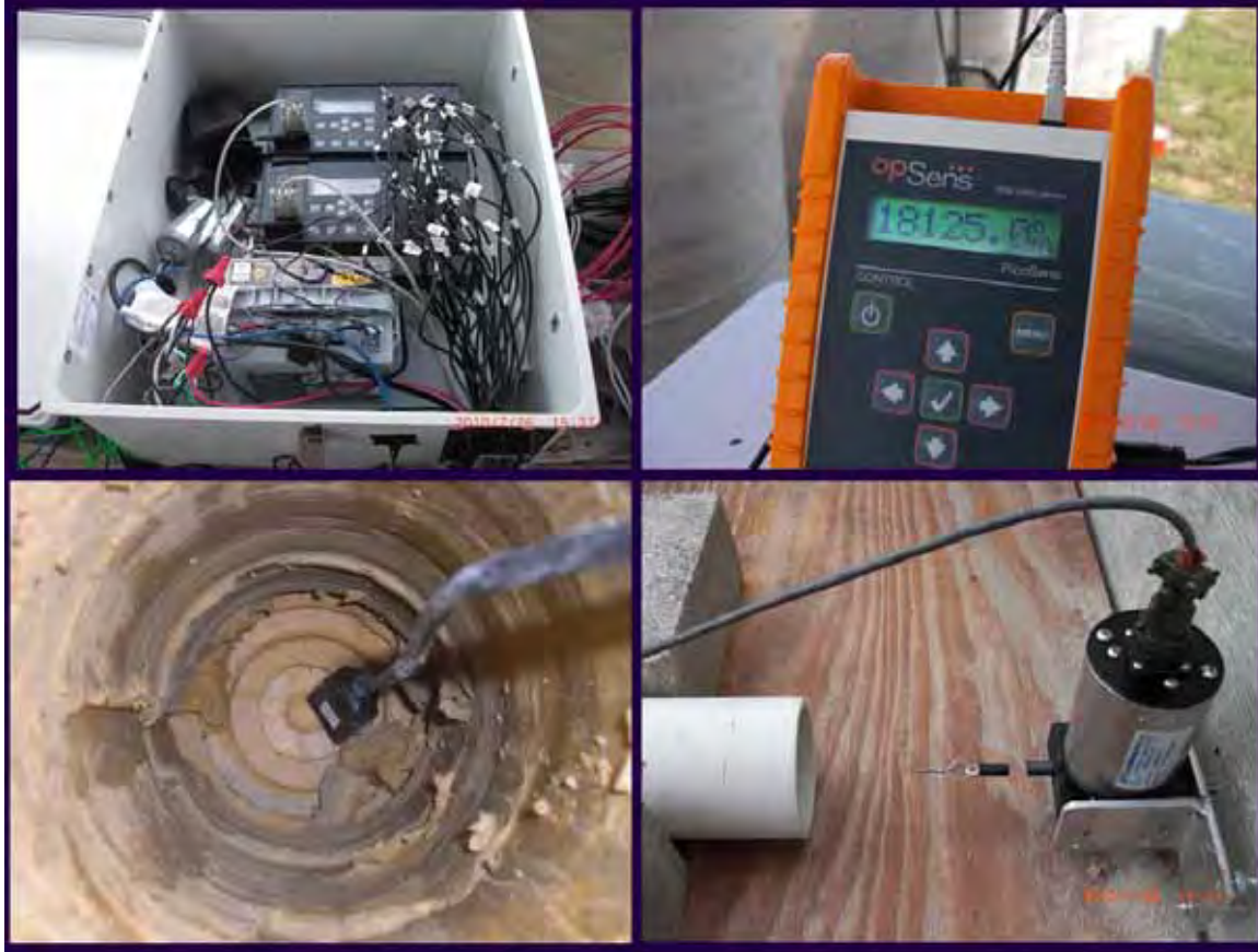
Figure 4.13: Instrumentation on the project site. Clockwise from top left: temperature resistant datalogger and enclosure for continuous strain readings; signal conditioner for individual strain readings; linear potentiometer; TDR probe installed through facing.
