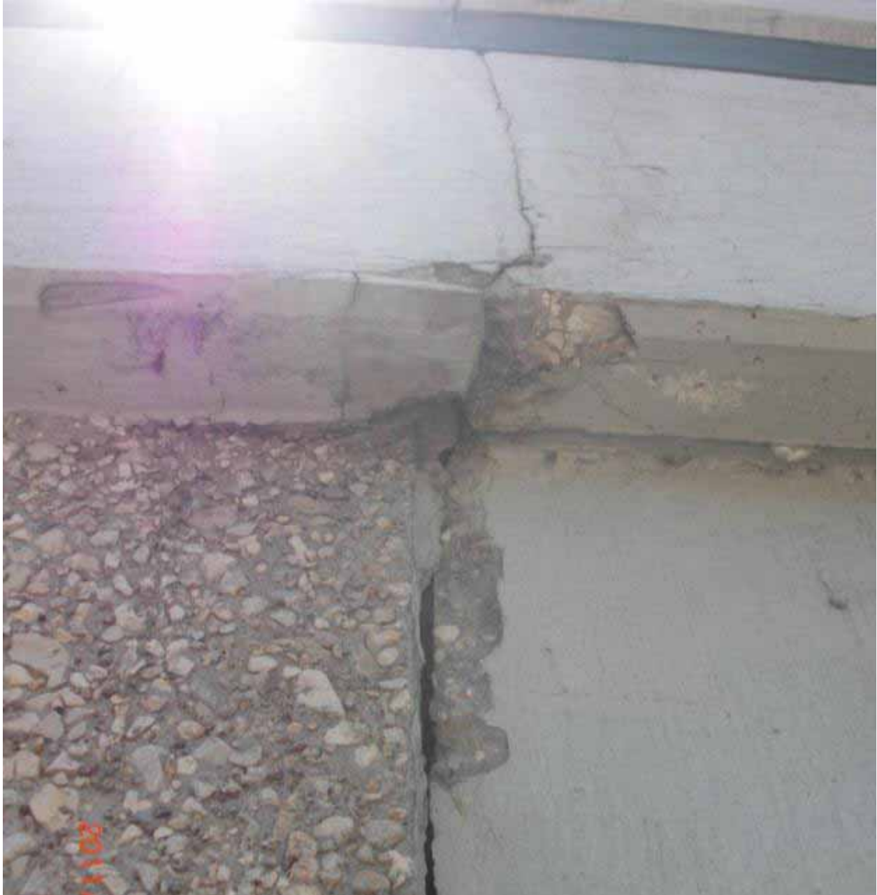
Figure 3.38: Some cracking was seen at the connection between two facing panels on the southwestern portion of the wall.
