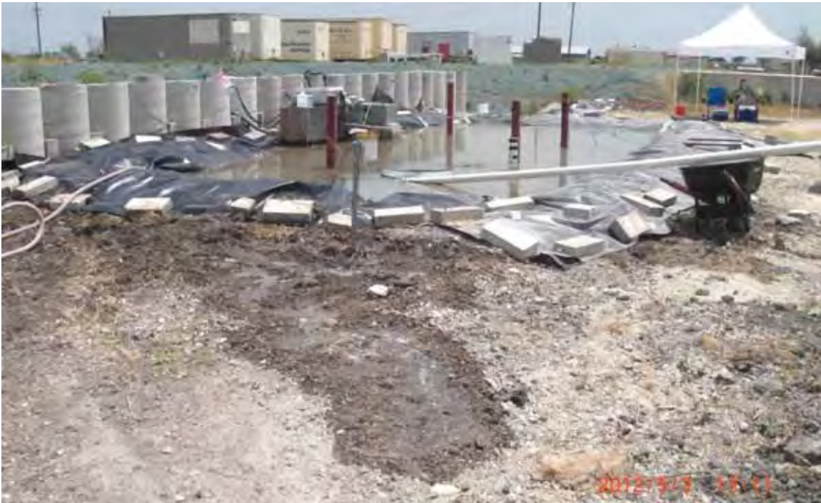
Figure 4.37: Leakage from west side of inundation zone.
