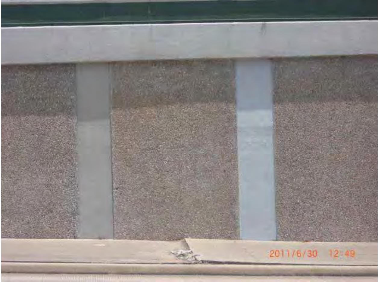
Figure 3.37: View of sidewalk damage along the base of the wall.
