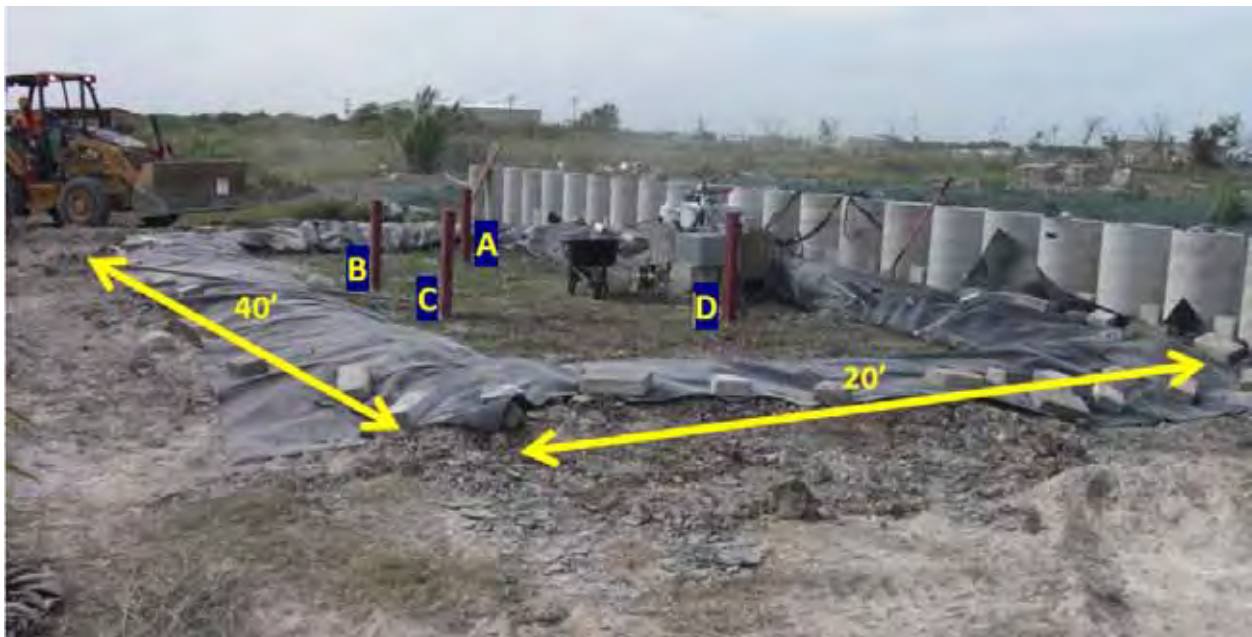
Figure 4.26: The four standpipe piezometers installed behind the wall in the inundation berm.
