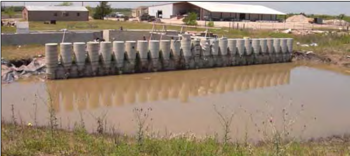
Figure 5.26: Flooding in response to a large storm before the May 6, 2013, data surveys. Water level in the excavation reached ground surface.
