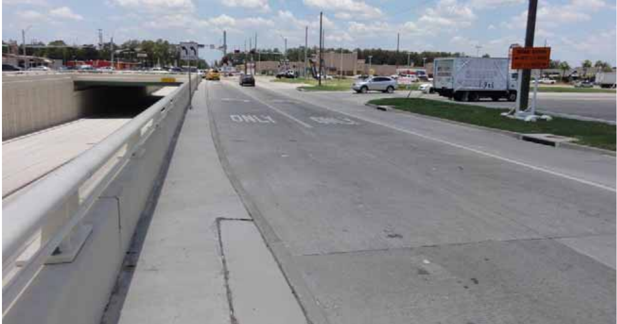
Figure 3.28: Paved area behind the wall. In all locations, pavement extends at least 30 feet behind the wall.
