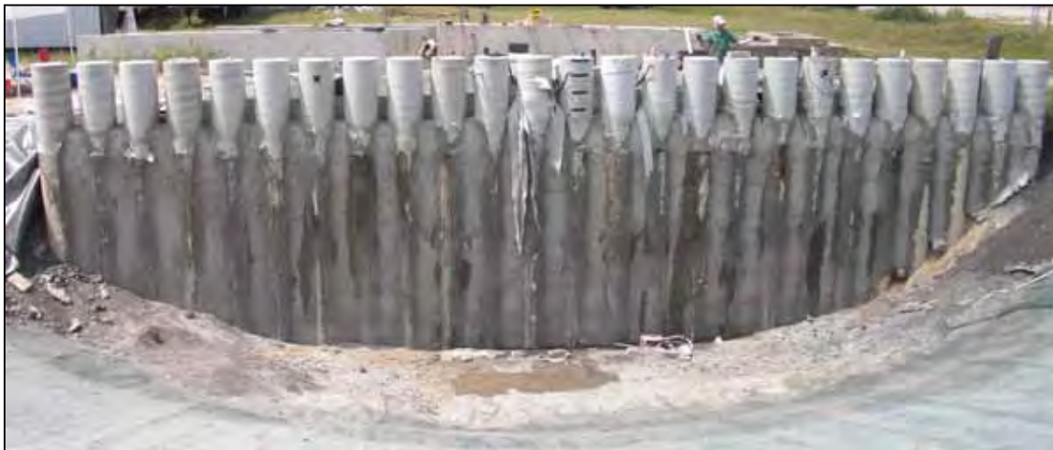
Figure 5.38: Water infiltration into the excavation was first observed 90 minutes from the start of inundation.
