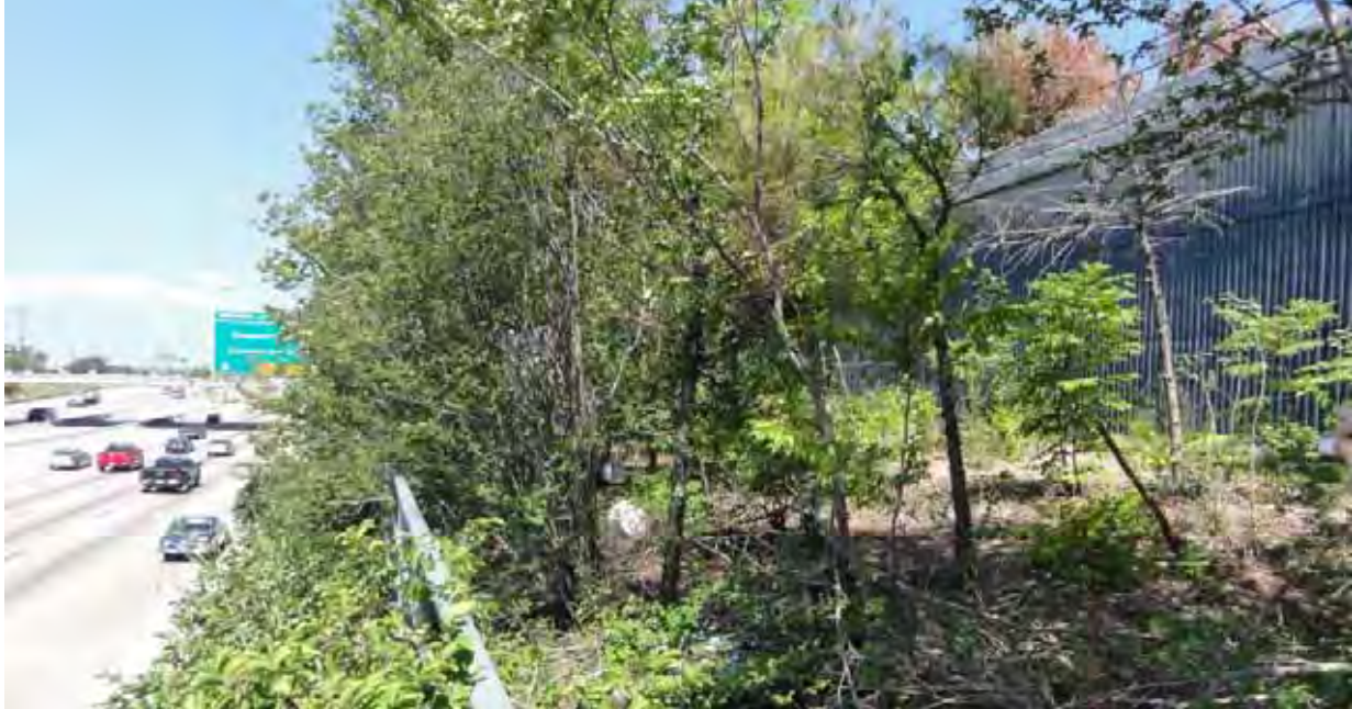
Figure 3.33: Approximately 40 feet of exposed soil behind the wall near Hazard Street (facing west).
