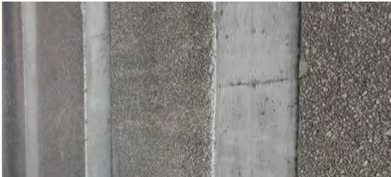
Figure 3.36: Example of imperfection in white concrete facing, possibly caused by a seam in the plywood formwork.
