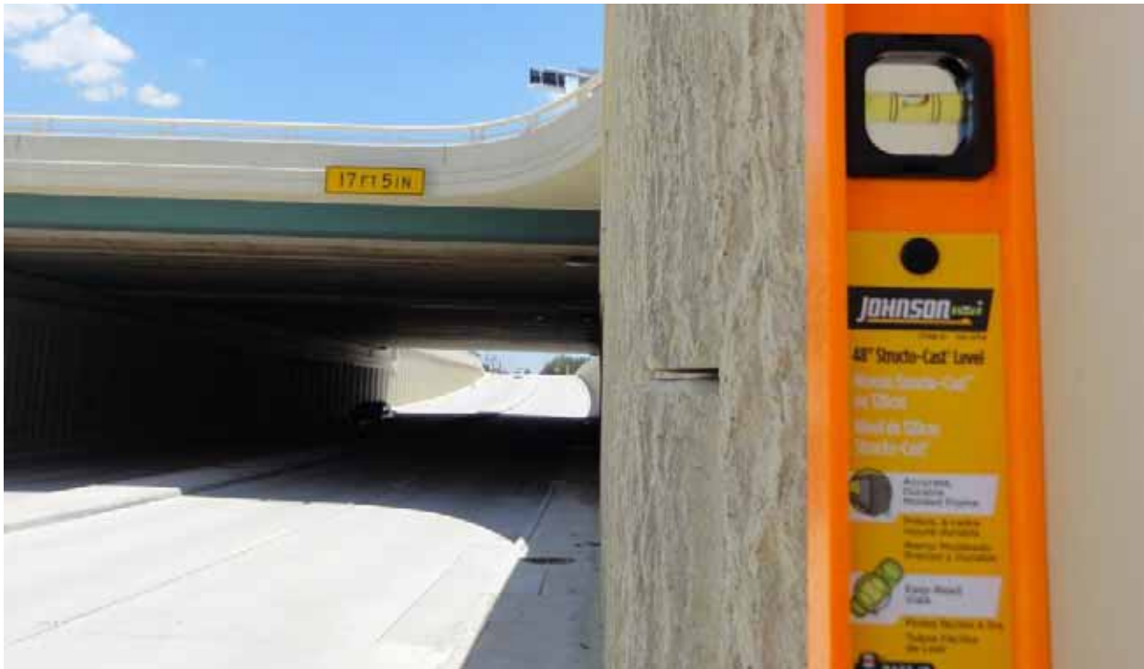
Figure 3.27: Wall facing was observed to be vertical and in good condition throughout the project area.
