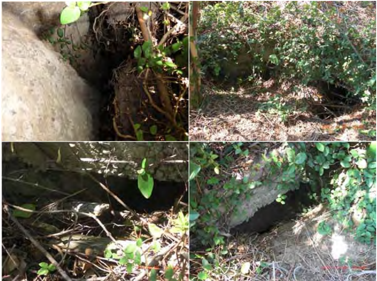
Figure 3.34: Several gaps were observed between the shafts and the soil behind the wall.
