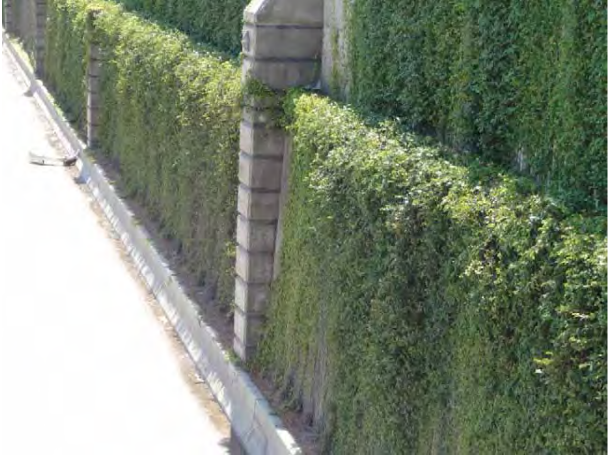
Figure 3.32: Dense vegetation and batter angle on concrete facing panels. Sound wall is located above main retaining structure.
