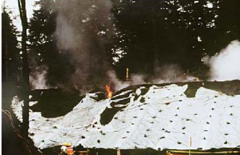
Figure 3.3: Removal of Tire Shred Section from Il Waco, Washington (Wappett 2004)
