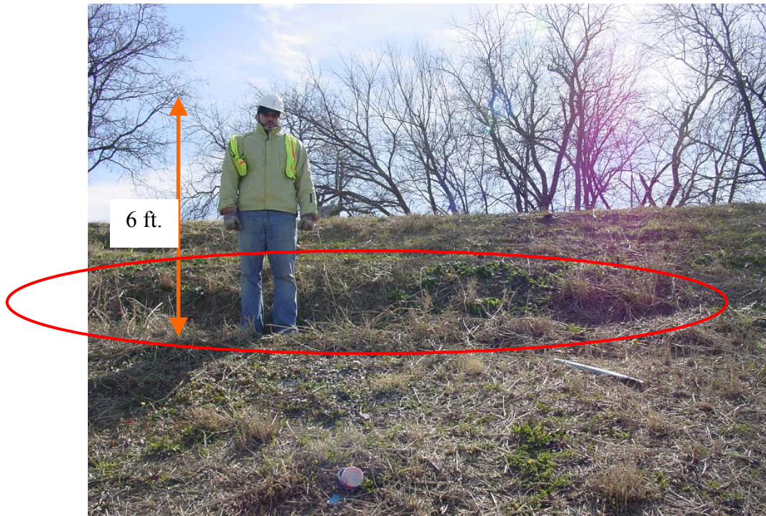
Figure 9.12: Soil Slump Observed at the Upper East Corner of the Tire Bale Slope
