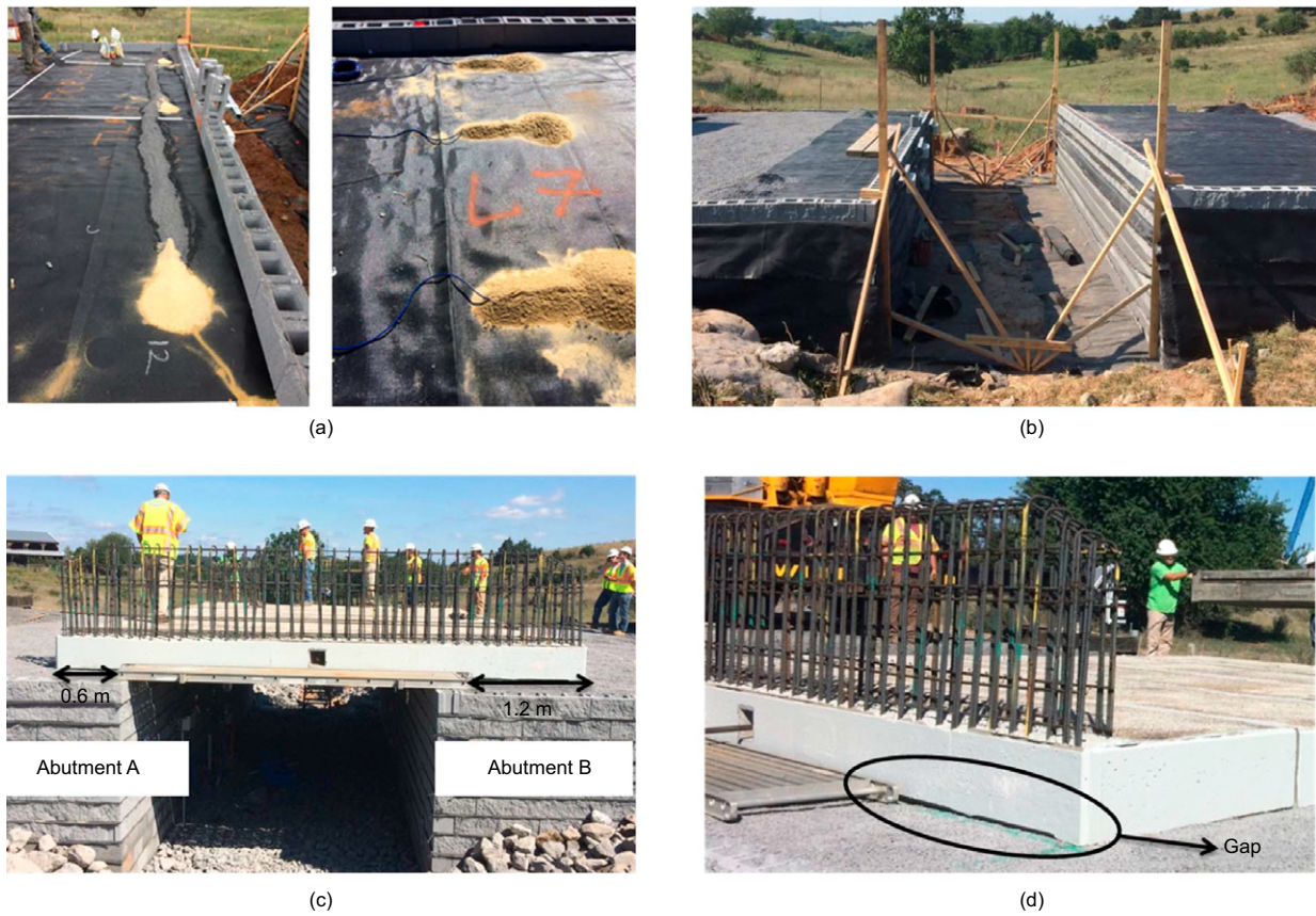
Figure 4. Details of the GRS-IBS constructed: (a) installation of EPCs; (b) placement of geotextile reinforcements; (c) placement of bridge slab; and (d) gap between the top of reinforced aggregate and bottom of bridge slab. Notes: Figure 4a shows the placement of EPCs at different layers, placed both perpendicular to and parallel with the facing blocks. Figure 4b shows the placement of shorter and longer geotextile reinforcements. These reinforcements are depicted in Figure 3 with dashed lines. Figure 4c shows the differences in beam seat in abutments A and B
