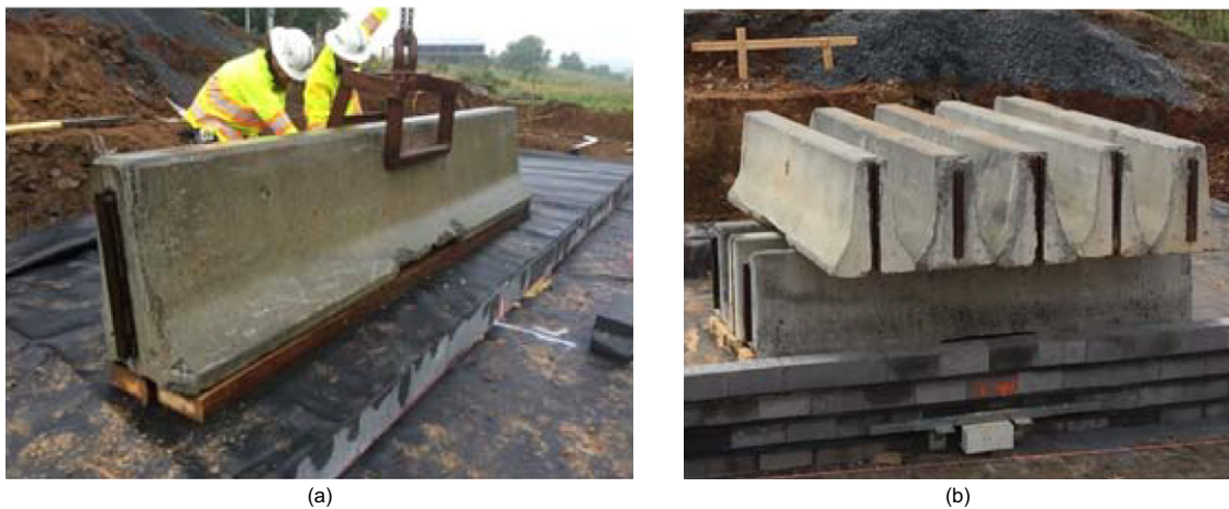
Figure 5. Placement of Jersey barriers along the facing of Abutment A to load the structure in stages: (a) single barrier; and (b) multiple barriers. Note: Locations of stage loading in different layers have been depicted in Figure 3a
