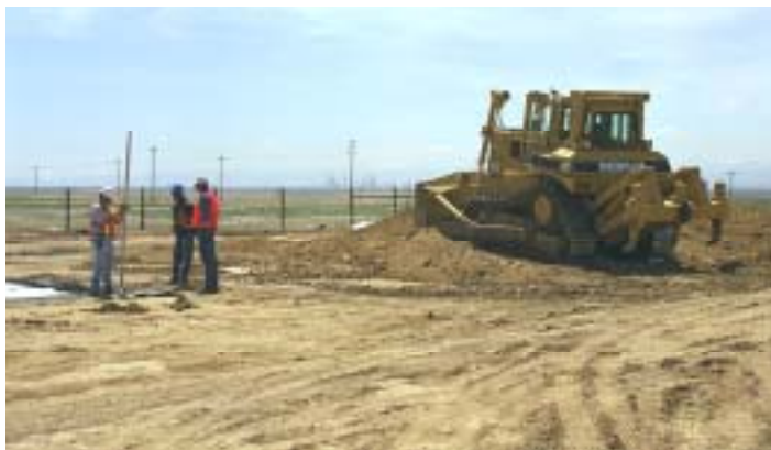
Figure 5-1. Placing soil lift for test pad construction at the Rocky Mountain Arsenal.
