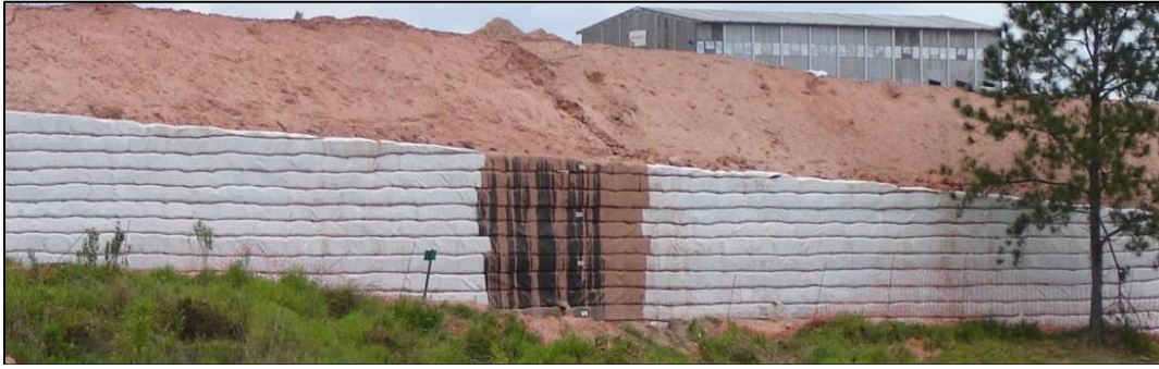
Figure 6 – View of geotextile reinforced soil walls during construction of the unreinforced embankment.
