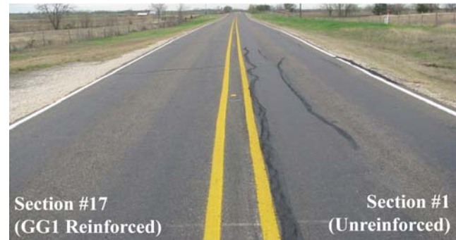
Fig. 8. Behaviour of unreinforced (Control) sections and geosynthetic reinforced sections over time (Survey #14 to #17).
