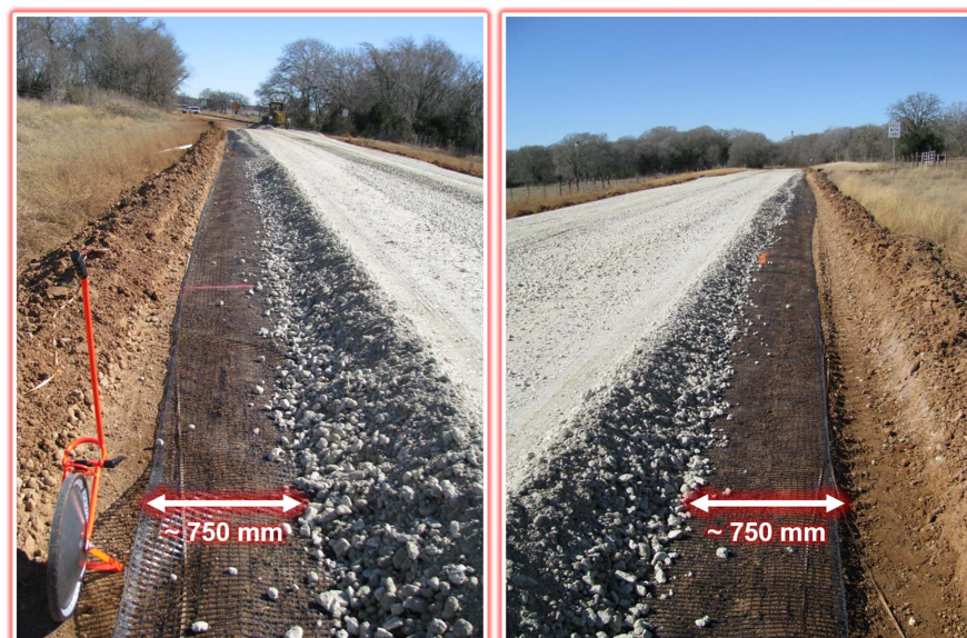
Fig. 4. Extent beyond road structural layers of geogrid in construction of the geosynthetic-stabilized base in FM1644.
