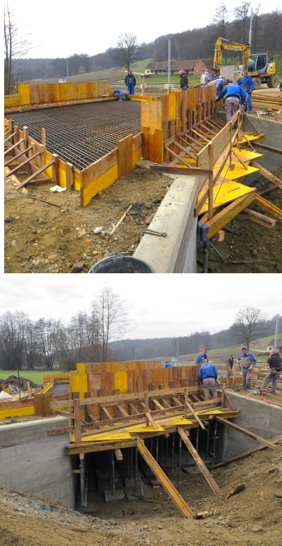
Figure 5: Formwork for cast-in-situ concrete of full height rigid (FHR) facings at the wall face
