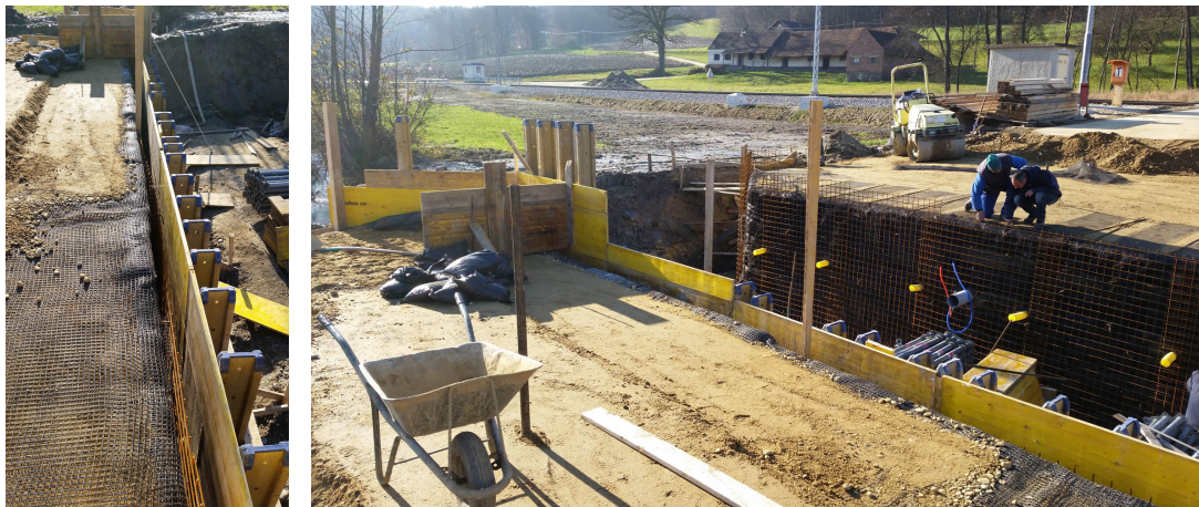
Figure 4: Formwork for cast-in-situ concrete of full height rigid (FHR) facings at the wall face
