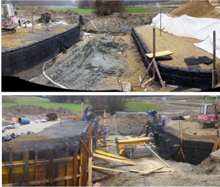
Figure 3: Construction of the GRS abutments by placing gravel bags on the shoulder of each layer and compaction of the backfill
