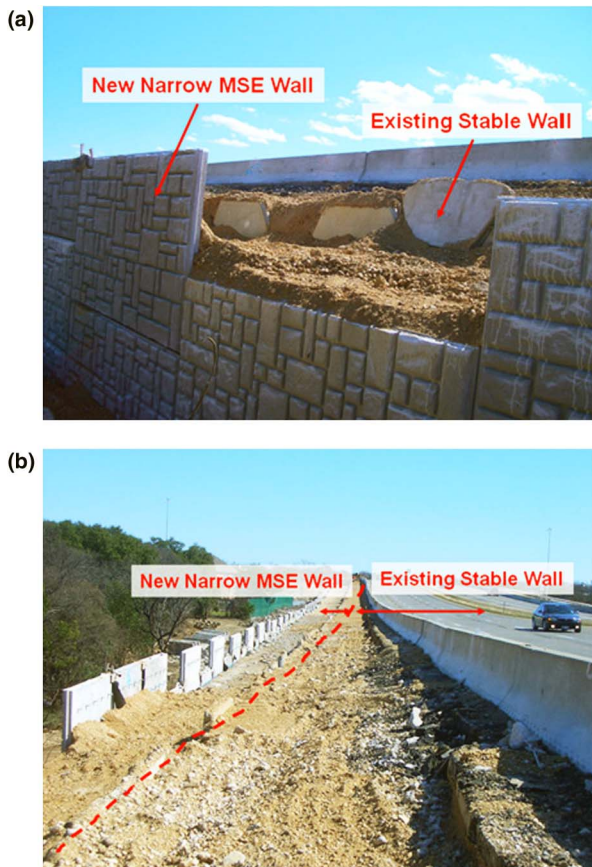
Fig. 2. Construction of a narrow MSE wall at Highway Loop 1 in Austin, Texas: (a) front view; (b) overview
