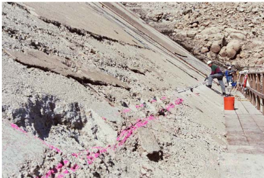
Figure 5. Typical section of the concrete face at Salt Springs Dam after 70 years of service and repairs.
