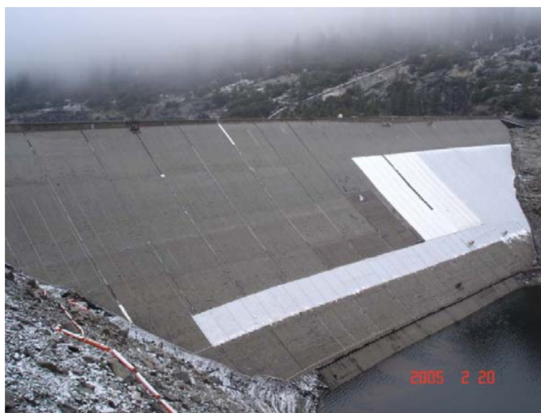
Figure 4. Installation of geomembrane at Salt Springs Dam, a CFRD dam in California.
