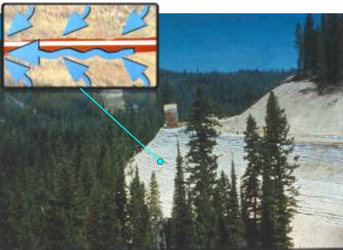
Fig. 10. Geosynthetic-reinforced slope in the Idaho National Forest, illustrating the use of reinforcement with in-plane drainage capabilities (Zornberg et al. 1997)
