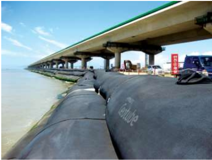
Fig. 6. Geotextile tubes for the construction of an artificial island at Incheon Grand Bridge Project, Korea (IFAI 2011)
