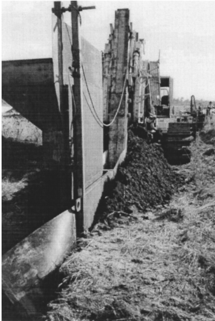
FIGURE 27.18 One pass trencher for installation of an HDPE vertical barrier system. (Photo courtesy of Groundwater Control, Inc.)
