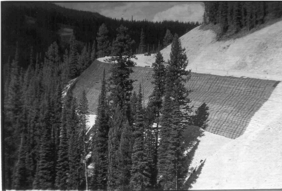
FIGURE 37.16 Erosion control mat placed to help establish the vegetation on the face of a 1H:1V reinforced soil slope.
