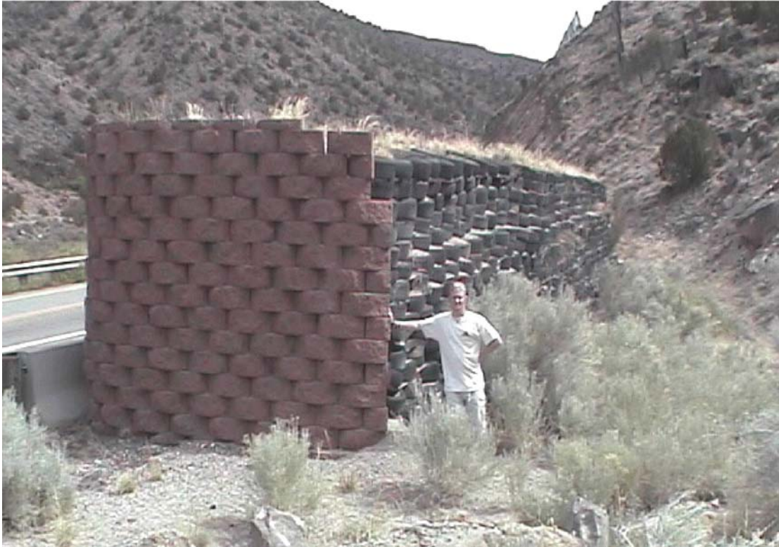
Figure 2.1 Geosynthetic reinforced soil (GRS) rockfall barrier with tire facing in New Mexico (Christopher, 2002)
