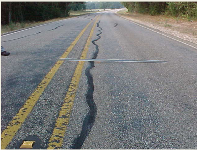
Figure 1. Typical longitudinal crack developed on pavements over expansive clays.
