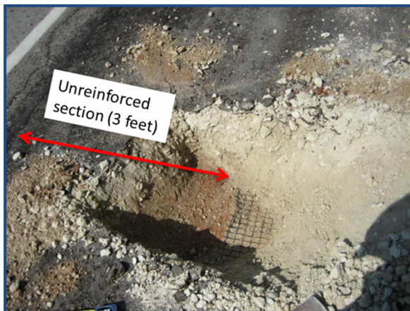
Figure 5. View of edge of geogrid reinforcement, directly underneath longitudinal crack.
