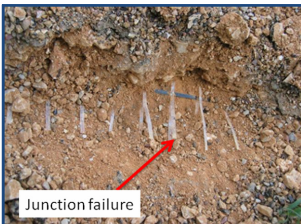
Figure 6. Separation of longitudinal and transverse ribs at junctions of Geogrid B at FM 1774
