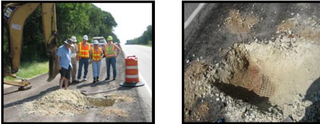
Figure 2 Longitudinal cracks in the unreinforced section of FM 542 pavement
