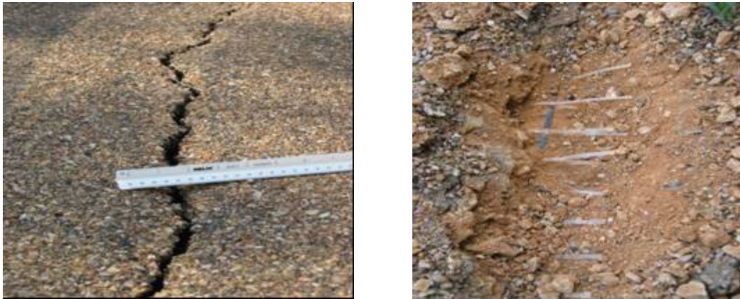
Figure 4.a) Longitudinal crack on the pavement reinforced with geogrid type 2 at FM 1774 (Bryan District) b) Slippage between longitudinal and transverse ribs at junction of geogrid type 2 at FM 1774 (Bryan District)
