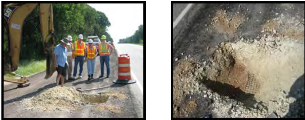
Figure 3.1: Longitudinal cracks in the unreinforced section of FM 542 pavement
