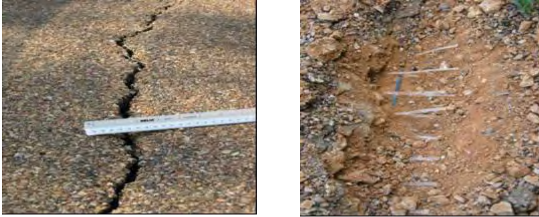
Figure 3.3: a) Longitudinal crack on the pavement reinforced with geogrid type 2 at FM 1774 (Bryan District) b) Slippage between longitudinal and transverse ribs at junction of geogrid type 2 at FM 1774 (Bryan District)
