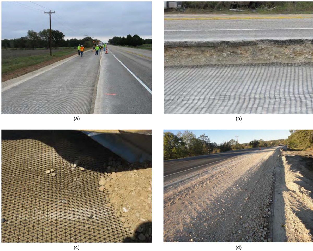
Figure 20. View of geosynthetic deployment during 2011 reconstruction of SH21 (Case Study D) (photos courtesy of TxDOT): (a) installation of biaxial geogrids; (b) view of old pavement layers; (c) installation of multiaxial geogrids; (d) widening of shoulders and construction of new base course
