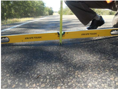
Fig. 3. Measurements of rutting in FM2 road test sections
