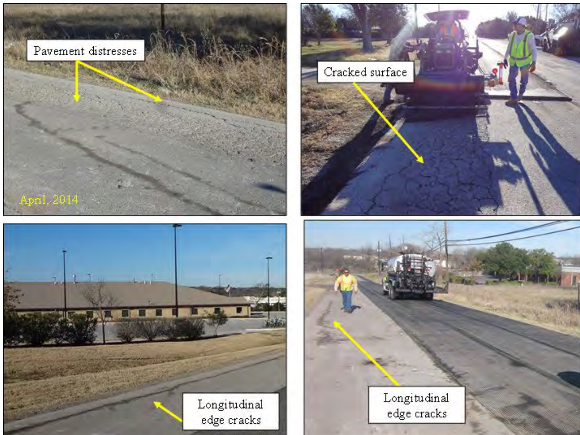
Figure 3. Distresses in the Pre-existing Roadway: April 2014.
