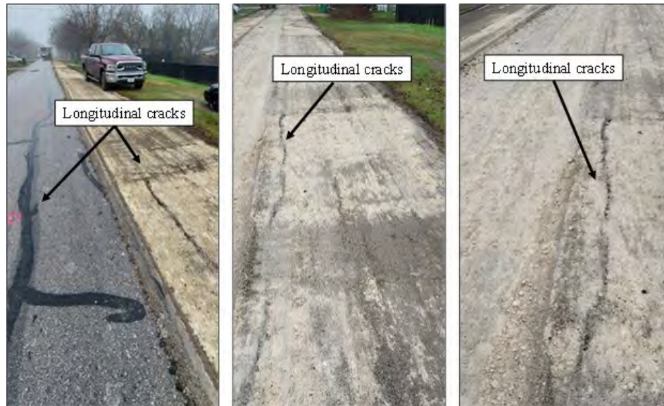
Figure 1. Examples of longitudinal cracks from expansive subgrades, in Taylor, Texas.
