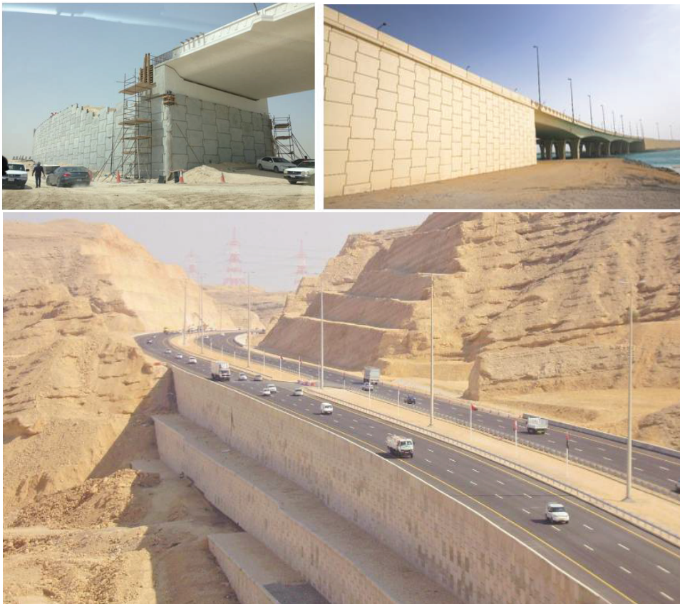
Fig. 2. Examples of polymeric strip reinforced soil walls and abutments in Middle East [7].
