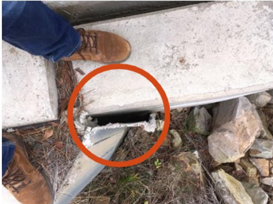
Figure 3. Gap formed between the wingwall and side of the abutment wall.
