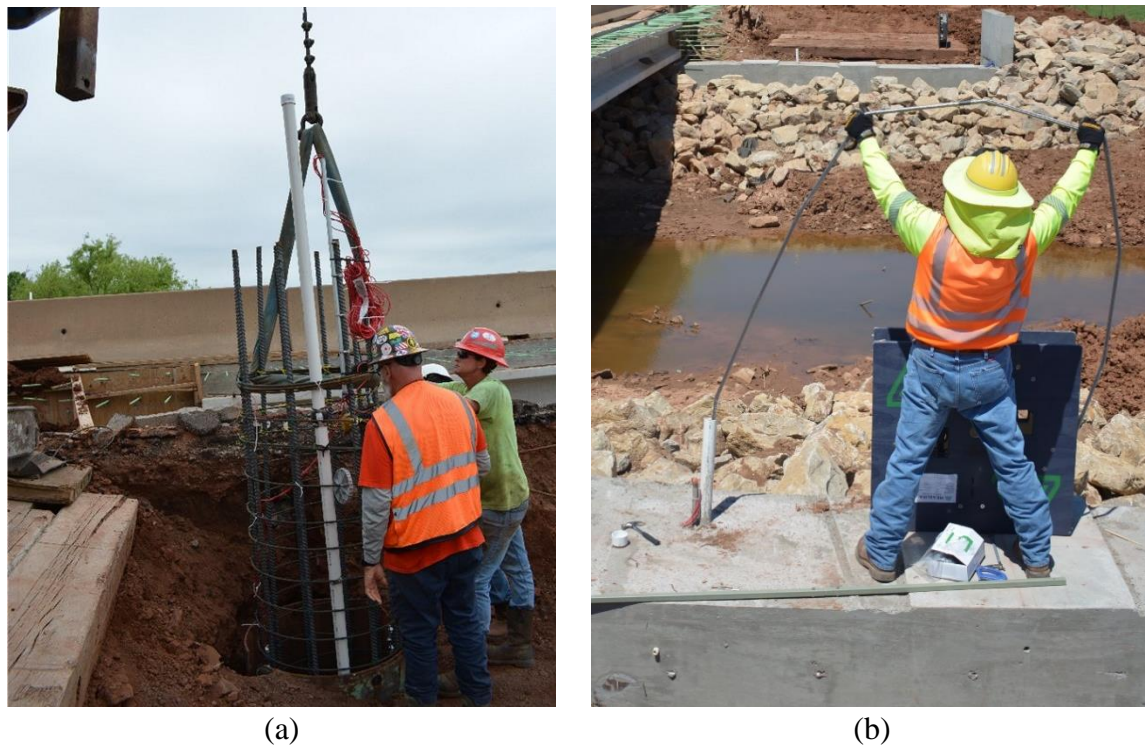
Figure 2. (a) Installation of the drilled shaft rebar cage fitted with a shape array casing (b) installation of shape array inside the casing after the abutment caps were formed
