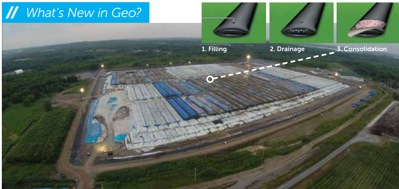
Figure 1. View of stacked geotextile tubes for containment of dredged sediments showing detail of multiple tube operation stages. (Photo courtesy of TenCate Geosynthetics.)
