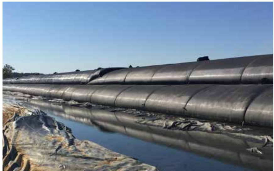
Figure 2. View of geotextile tube wall filled with re-used fly ash in an ash pond at a Mid-Atlantic utility site. (Photo courtesy of TenCate Geosynthetics.)
