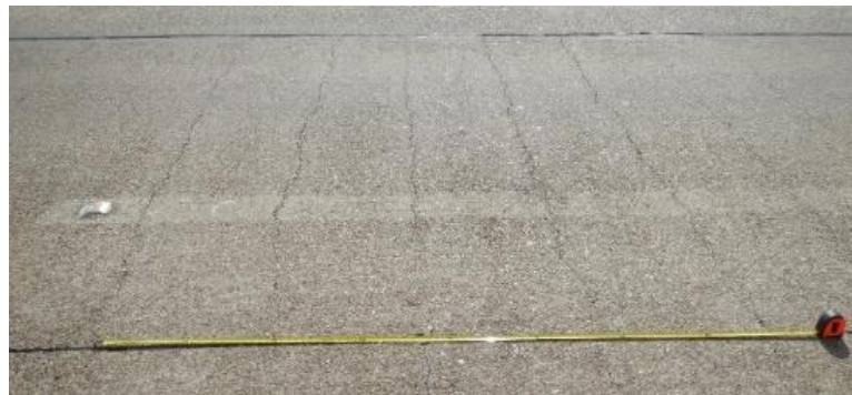
Figure 2.11: CRCP with well-controlled transverse cracks in US 347 (Won, 2021).
