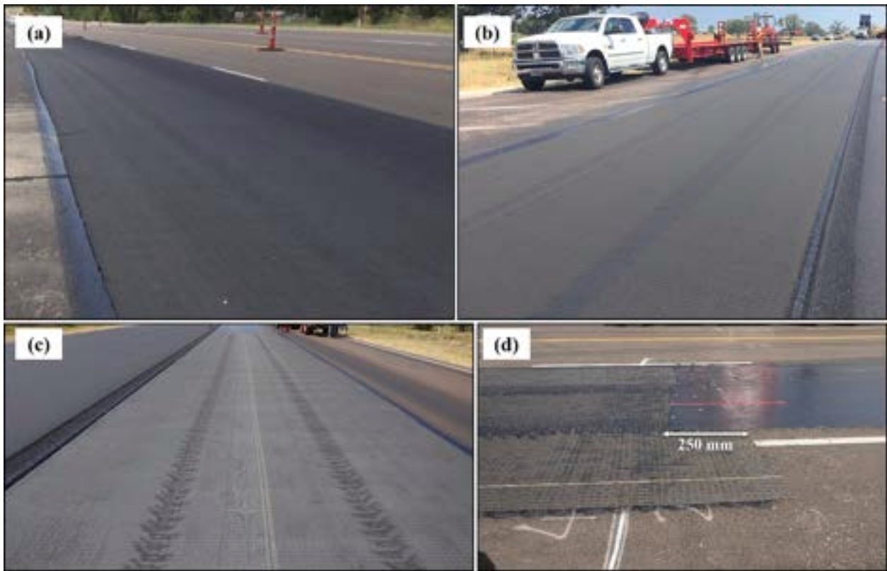
Fig. 10. Photos showing proficient geosynthetic installation in experimental test sections: (a) GS-1; (b) GS-2; (c) GS-3; and (d) overlap between geosynthetics GS-6 and GS-8 in longitudinal direction.
