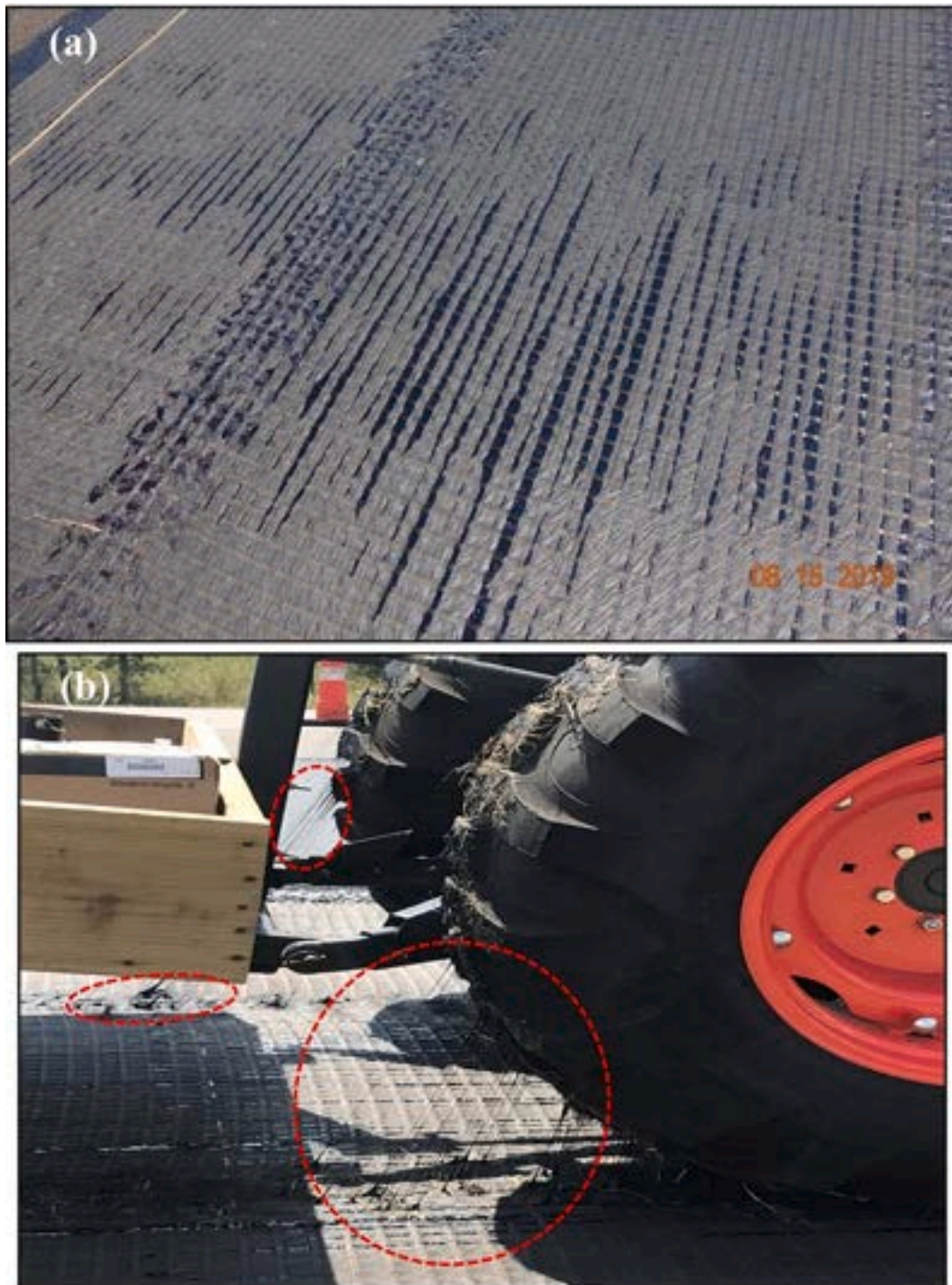
Fig. 12. Influence of temperature on tack coat and geosynthetics: (a) blistering of geotextile backing; and (b) tracking of geosynthetic installation tractor wheels.
