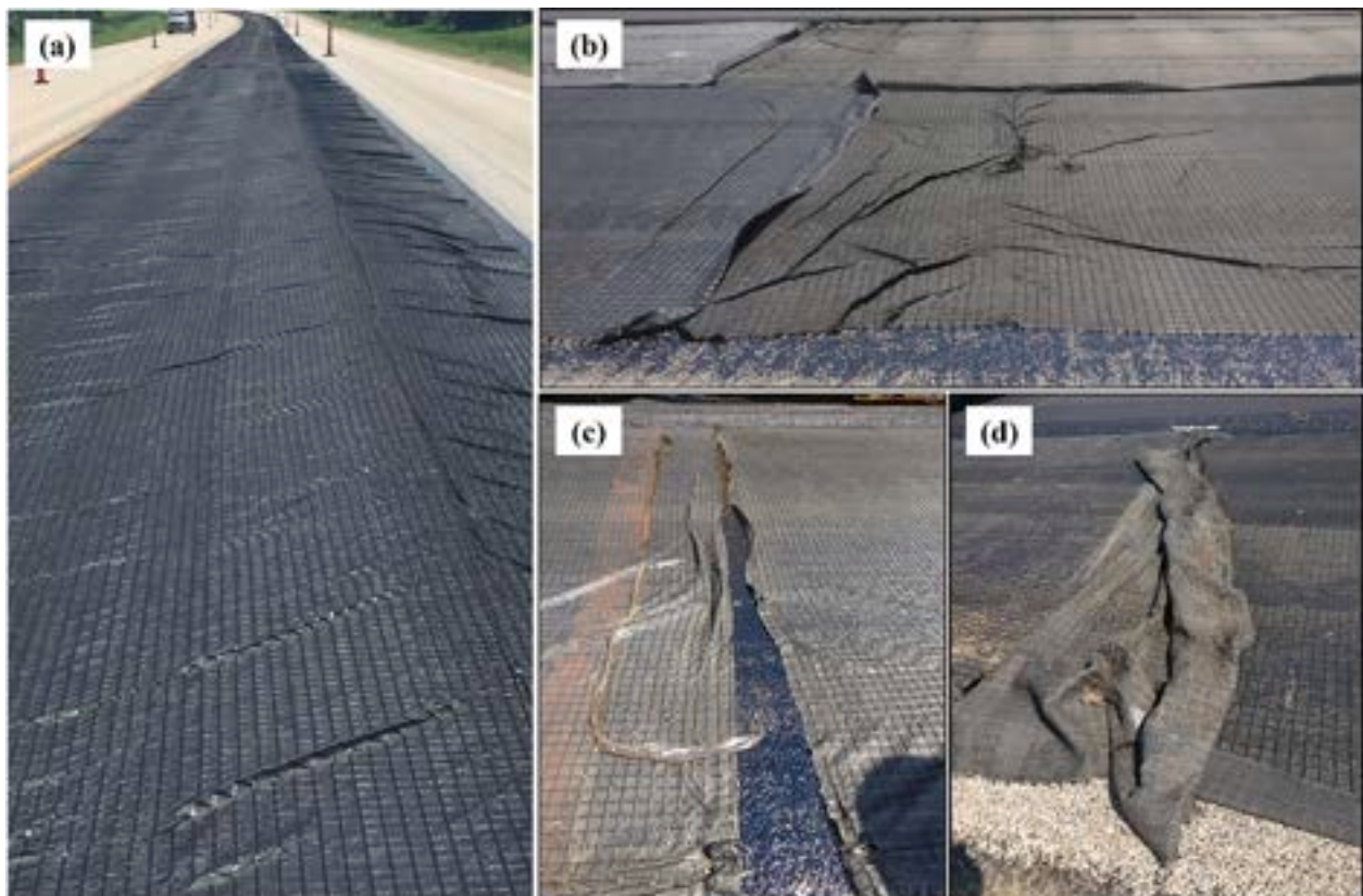
Fig. 11. Photos showing poor geosynthetic installation: (a) numerous wrinkles along roadway; (b) inadequate geosynthetic overlap in longitudinal and transverse directions; (c) no geosynthetic overlap in longitudinal direction; and (d) excess geosynthetic overlap in longitudinal direction.
