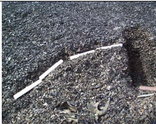
Photo A-24: Protection of Wiring of Instrumentation in the Large Tire Shred-Only Stockpile
