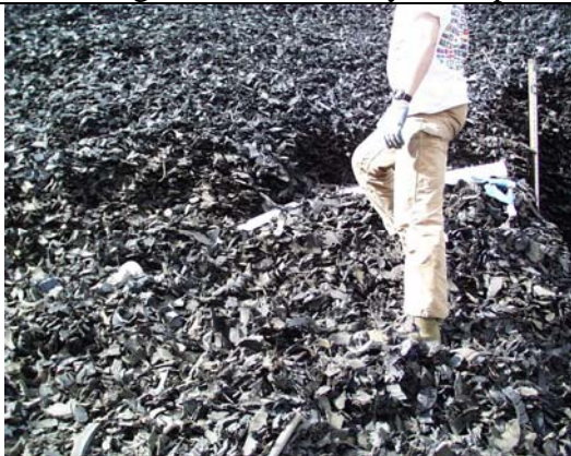
Photo A-29: Closure of the Ditch Excavated for PVC Protecting Wiring of Instrumentation in the Large Tire Shred-Only Stockpile
