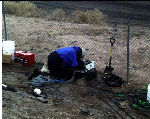
Photo A-11: Installation of Data logger and Multiplexer
