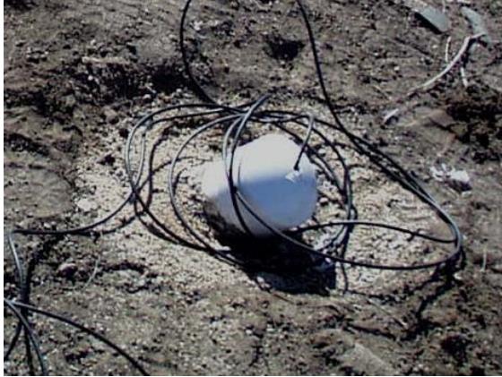
Photo A-7: Detail of Bentonite Seal
