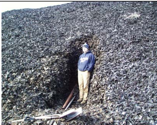
Photo A-23: Front View of Ditch in Large Tire Shred-Only Stockpile Excavated for Installation of Instrumentation
