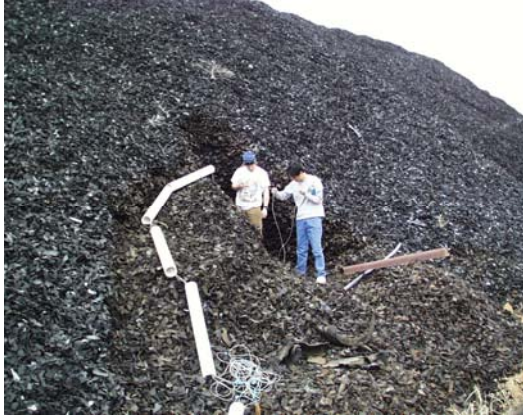
Photo A-25: Installation of Wiring for Instrumentation of the Large Tire Shred-Only Stockpile
