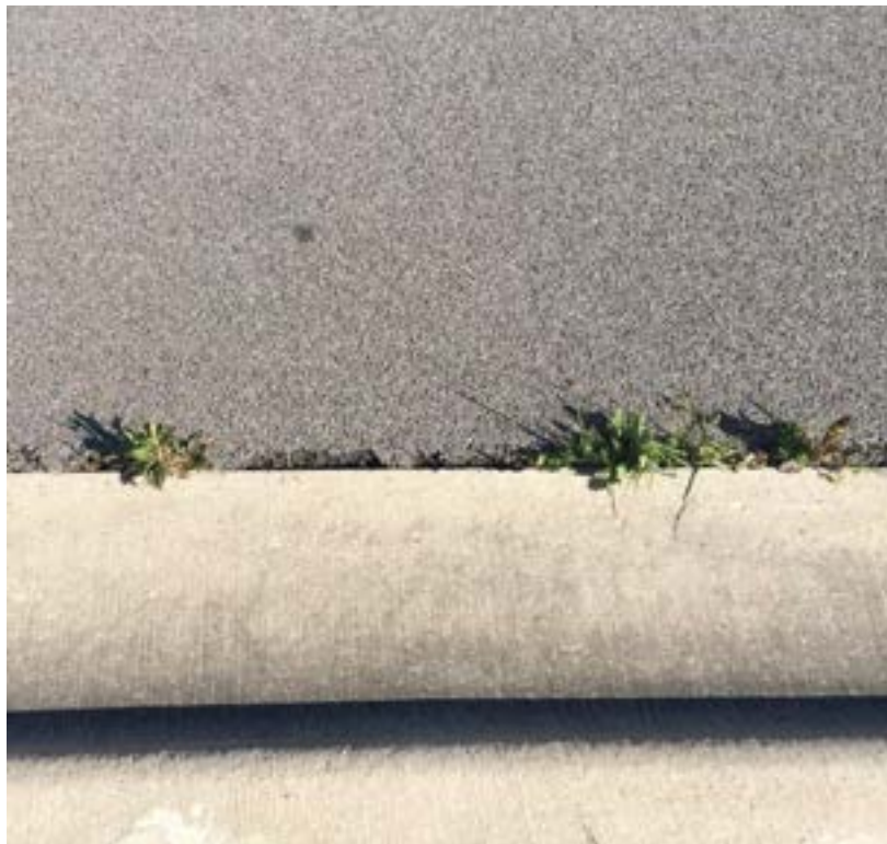
Figure 4.94: Gap between Curb and Asphalt at Site 6
