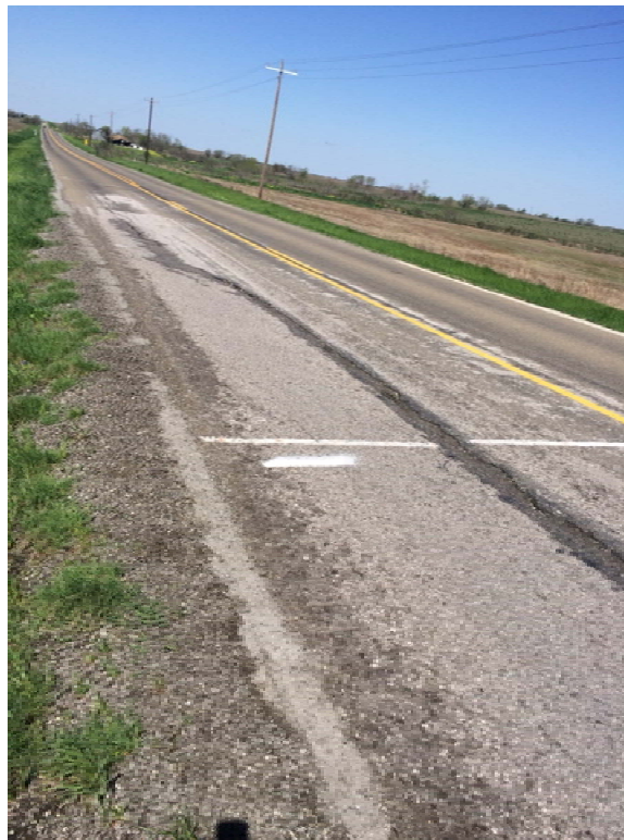
Figure 5.55: Longitudinal Crack at FM 972
