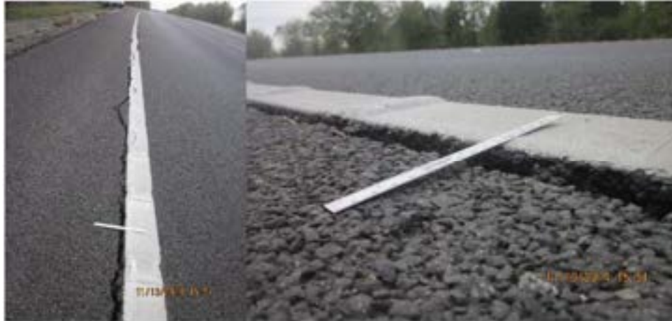
Figure 4.132: Edge Cracking at SH-21 (Garcia 2015)
