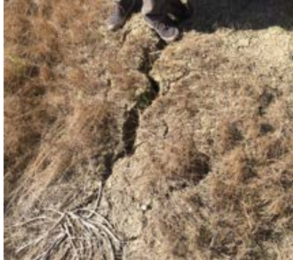
Figure 4.18: Cracking of Heiden Clay near La Frontera Blvd
