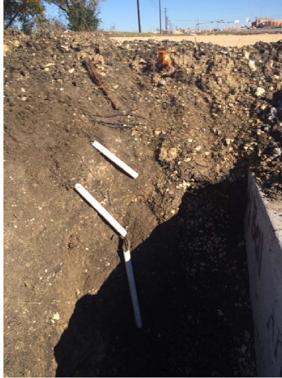
Figure 5.44: Installed Sensors at FM 685
